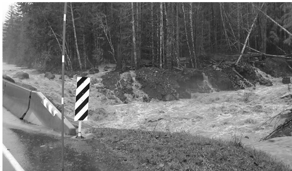
FIGURE 6. Heavy flood waters from Kautz Creek entering road culverts along Nisqually Road at Mount Rainier National Park (WA) during November 2008 flood.
