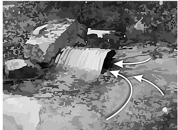
FIGURE 5. Culvert opening nearly submerged with heavy runoff entering the opening, which creates powerful suction and a hazard to anyone positioned in front of such an opening.
